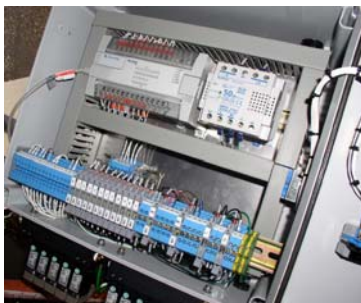
PROCESS LOGIC CONTROLLER
